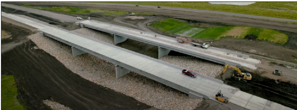
The I-29 construction as part of the Fargo-Moorhead Metropolitan Area Flood Risk Management Project. Photo courtesy of the FM Area Diversion
