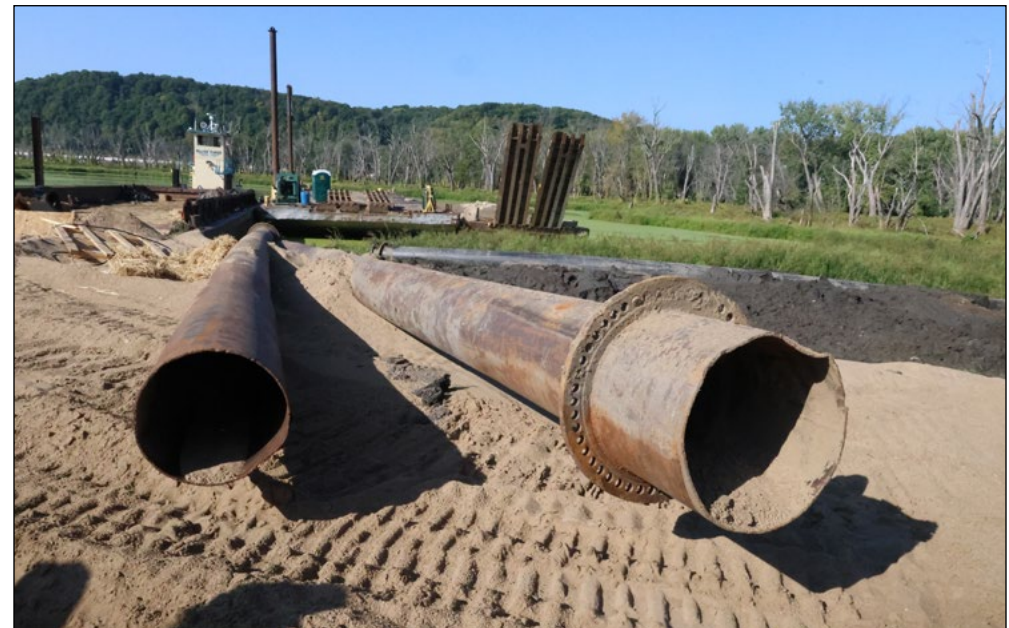
Construction is ongoing at McGregor Lake Habitat Rehabilitation and Enhancement Project, near Prairie du Chien, Wisconsin, Sept. 14. USACE St. Paul District photo by Melanie Peterson
