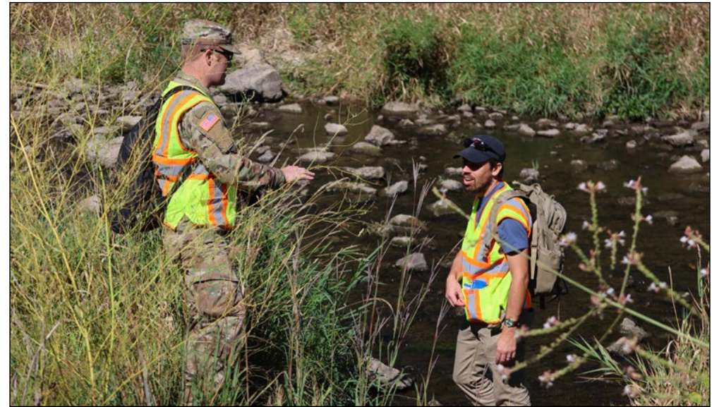
(left to right) Maj. John Walleser, geotechnical engineer, and Mike DeMars, structural engineer, inspect a flood risk management channel in Rochester, Minnesota, Aug. 31. USACE St. Paul District photo by Elizabeth Stoeckmann
