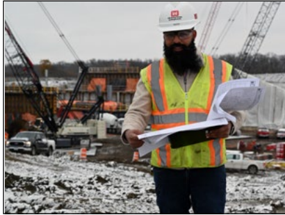
(cover) Sanjay Bimali, civil engineer, stands at the Diversion Inlet Structure, near Horace, North Dakota, Oct. 27. USACE St. Paul District photo by Patrick Moes
